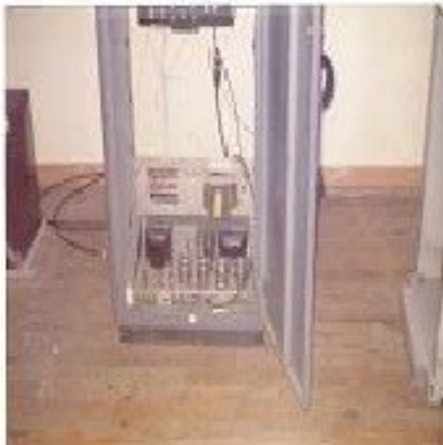
Fig 2: Bottom of the cabinet
